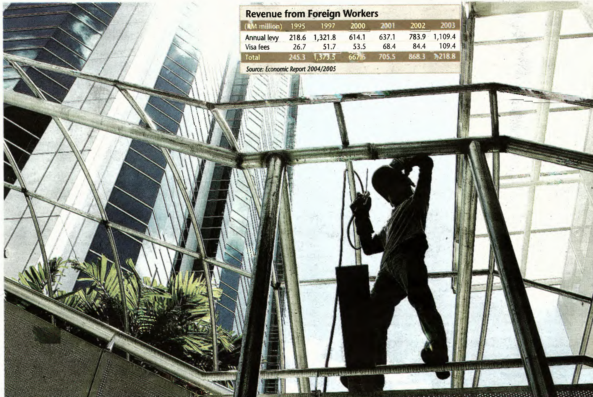
A welder working on the joints of a steel structure in Kuala Lumpur. Experts agree that Malaysia needs a long-term policy on foreign labour to provide clear road map on the recruitment of foreign workers.
